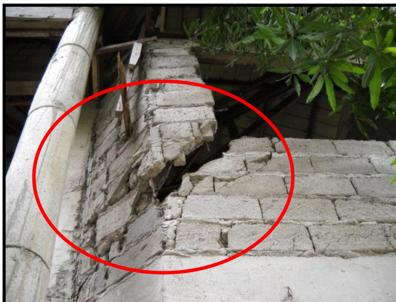
Plate No. 10 Dislocated wall section due to lateral movement of fault in Tunasan, Muntinlupa City.
