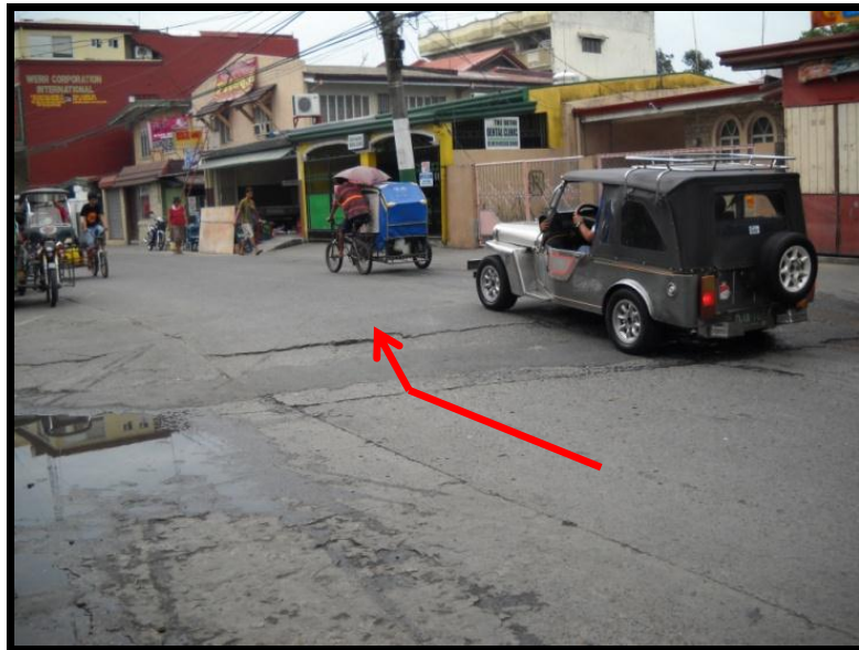
Plate No. 9 Vertical displacement reflected on road pavement in Tunasan, Muntinlupa City.
